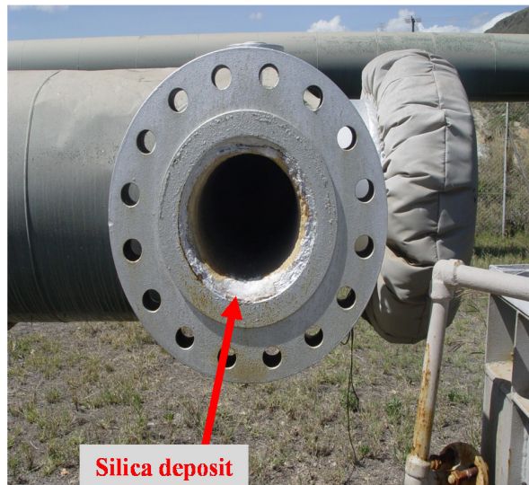
FIGURE 3: Silica scale forming in a steam delivery line. (Photo courtesy James Wambugu)
