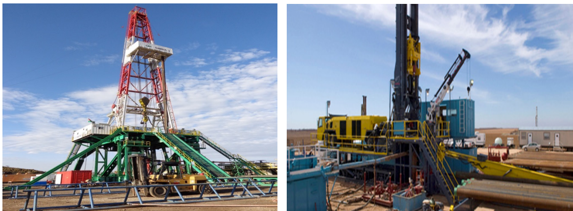
FIGURE 6a and 6b: 2000HP land rig and Atlas Copco predator rigs used at Menengai
