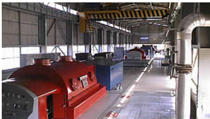
FIGURE 7: Machinery room in Ahuachapan power plant
