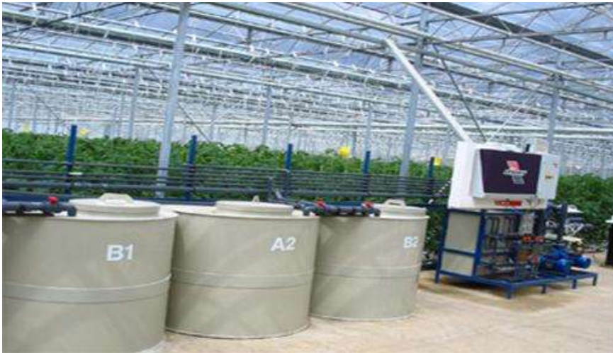
Greenhouse heating – Livada, Bihor County
