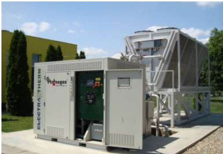
50 kWe Binary Cycle ORC Geothermal Power Plant installed in Oradea by Transgex Company
