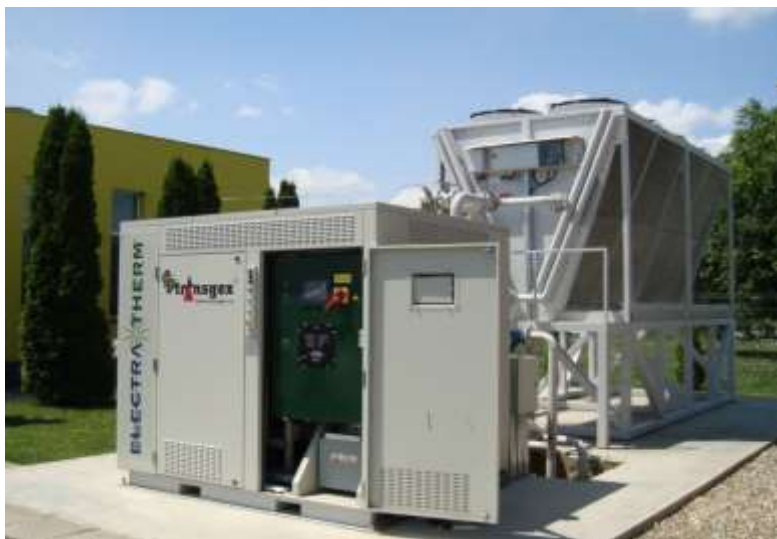
50 kW Binary Cycle ORC Geothermal Power Plant installed in Oradea by Transgex Company
