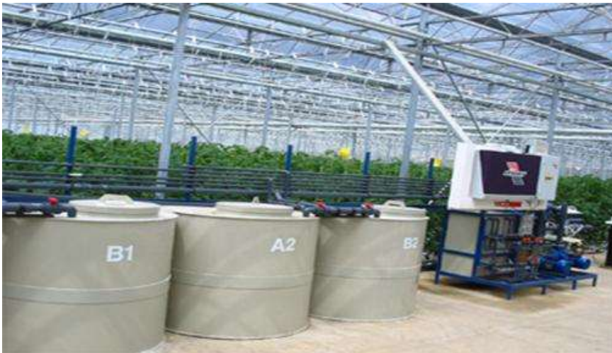
Greenhouse heating – Livada, Bihor County
