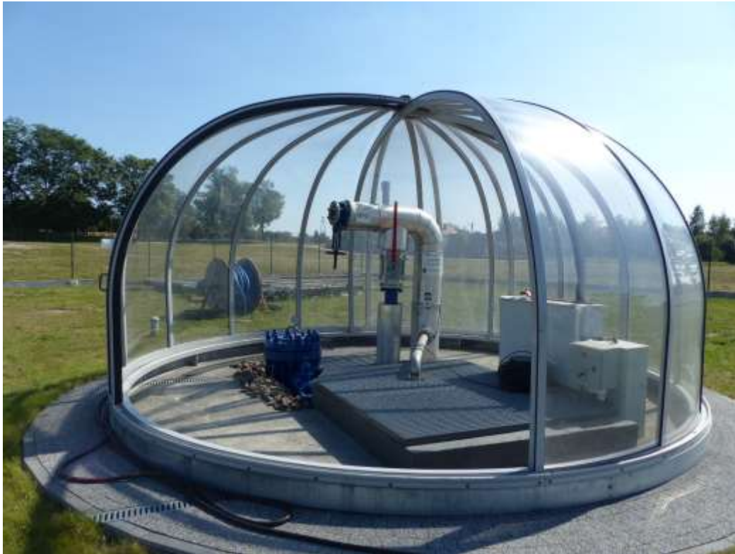
Fig. 2.30. Production well Poddębice GT-2, well head and connection piping
