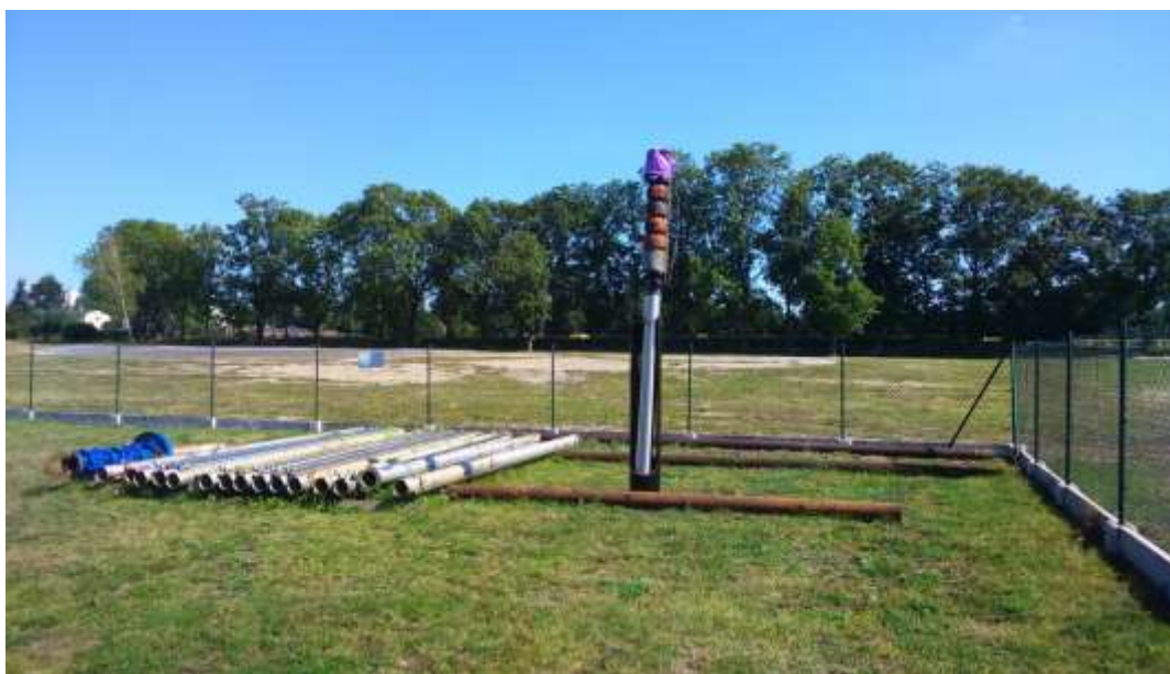
Fig. 2.31. Well pump from Poddębice GT-2 and pressure pipes
