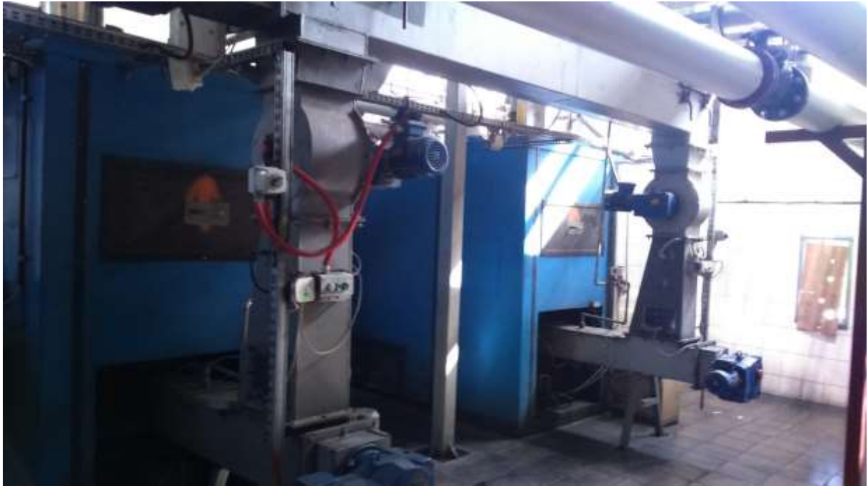
Fig. 2.38. Biomass peak load boiler station – district heating boilers
