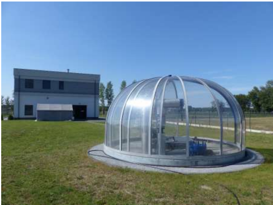
Fig. 2.16. Geothermal well head (Poddębice GT-2)
