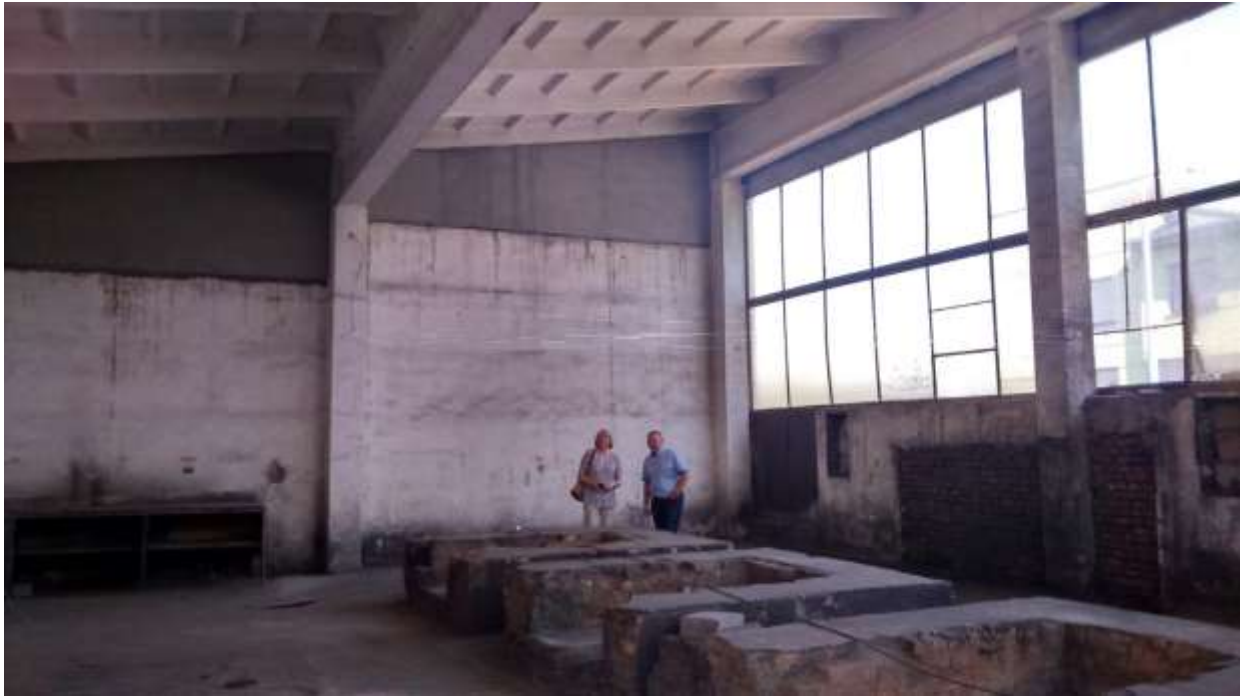
Fig. 2.40. Decommissioned coal fired peak load station in district heating system
