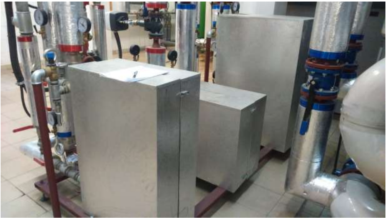
Fig. 2.41. Heating centre at Poddebice Health Center
