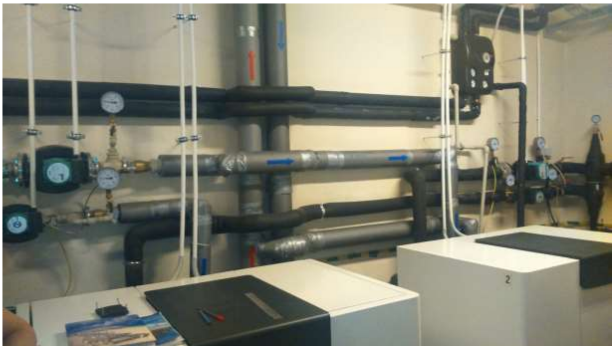
Fig. 2.42. Heat pumps at Poddebice Sports Centre
