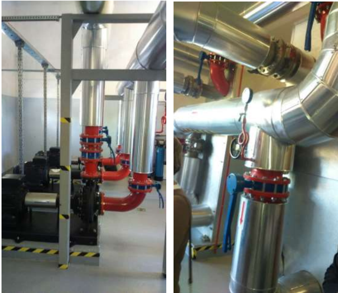
Fig. 2.33. Poddębice heat central, circulation pumps (left) and heat exchangers (right)
