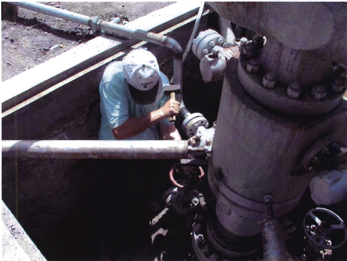
Figure 11. Bolts being tightened on the expansion spool of BO-2 (lower flange) where there was a leak (see Fig. 10).
