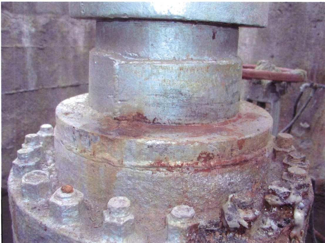
Figure 2. Photograph of leak area on BO-2 when I arrived. The leak had stopped due to self-sealing when the wellhead temperature dropped and thus the annular pressure.
