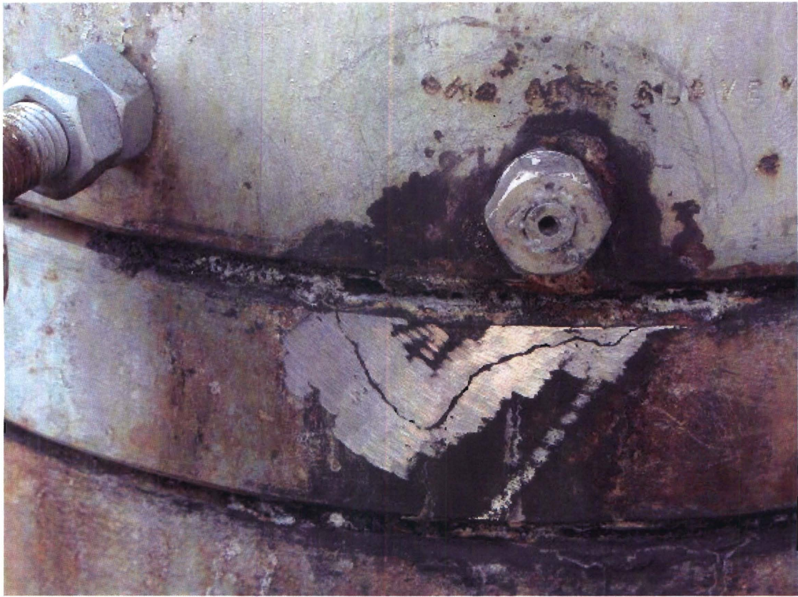
Figure 15. From under the scale deposits on the expansion spool a crack showed up on the flange just below the pressure release port. If it propagates deep it could result in leak.
