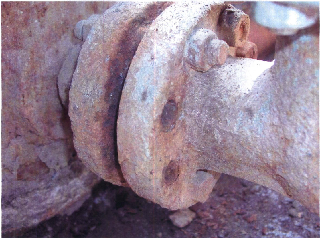
Figure 13. Close-up of bolts missing from flange on 13-3/8" casing head.
