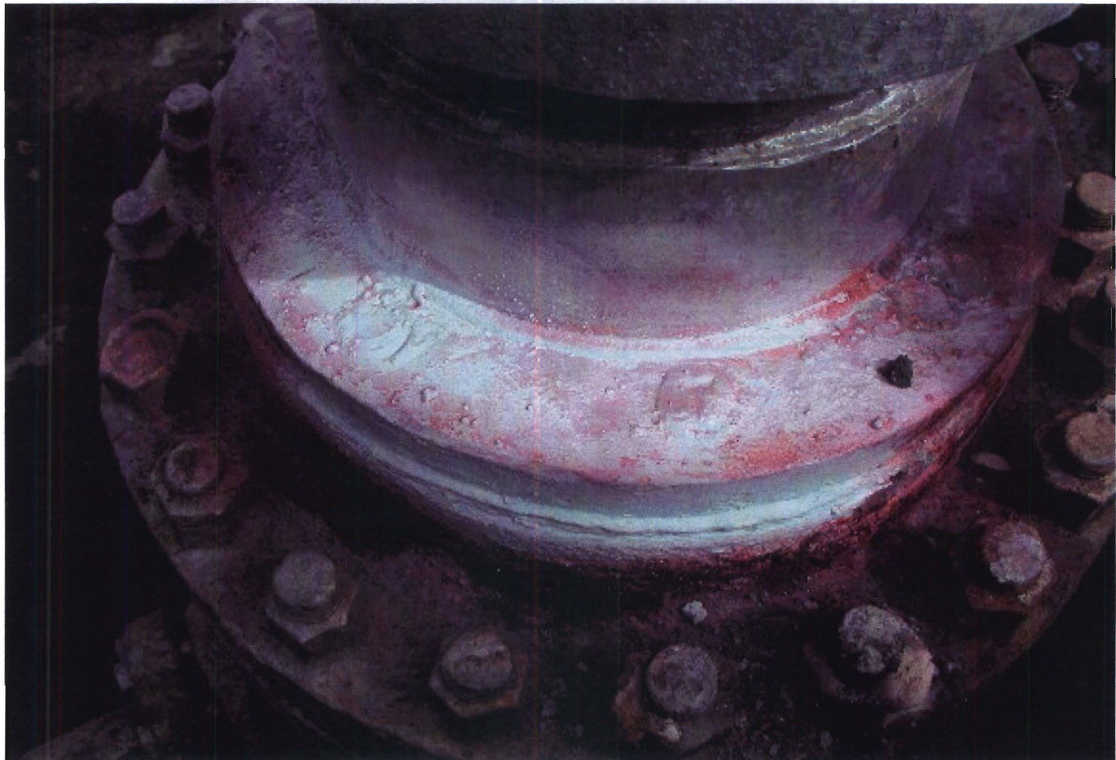
Figure 6. Die penetrant applied to welds on the wellhead of BO-2 where the leak occurred to identify cracks or holes. No welding cracks were detected, but a small pinhole in the weld covering one bolt hole showed up.
