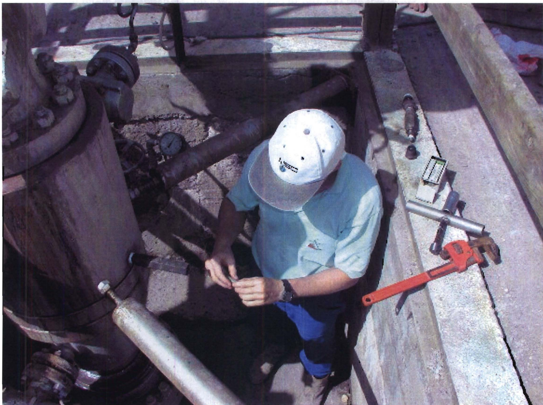
Figure 9. Expansion spool being repacked by Bernard. Injection tool is connected to the spool and he is holding the “rat shit”.
