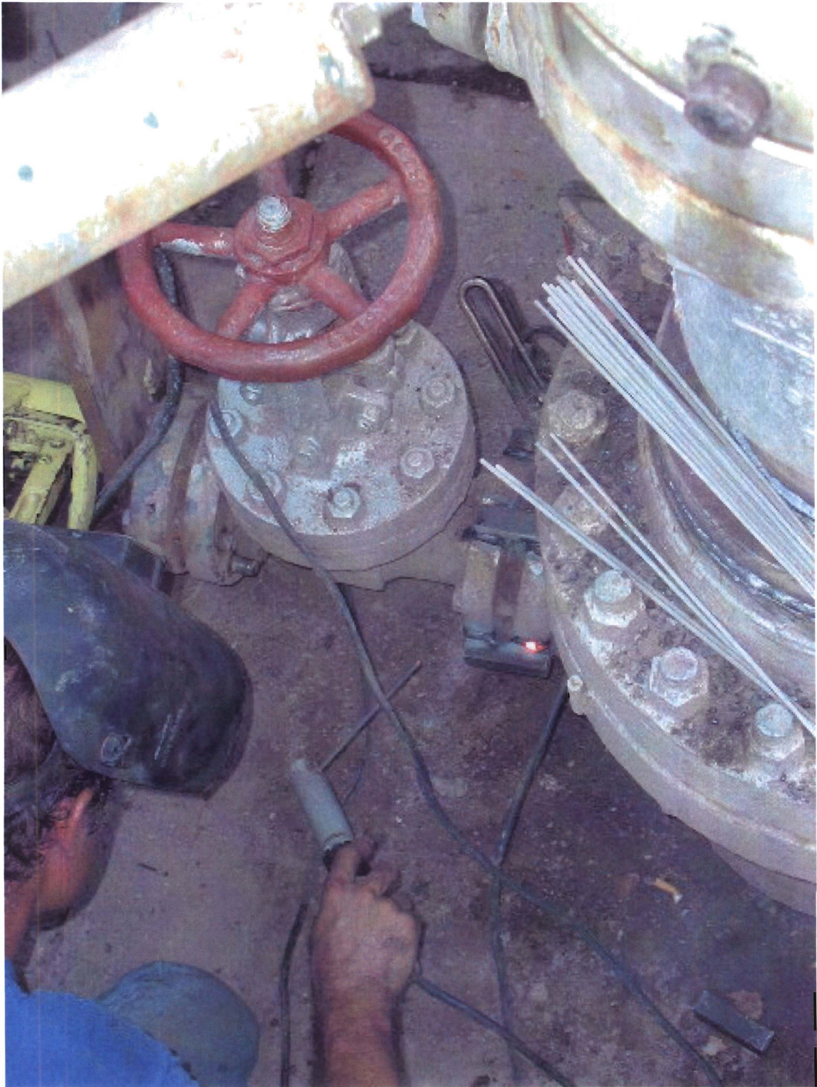
Figure 14. Reinforcing rods 20x20 mm welded over the flange pair of the 3-3/8" wing valve to make up for the loss of the two corroded bolts and suspected weakness of the other stud bolts.
